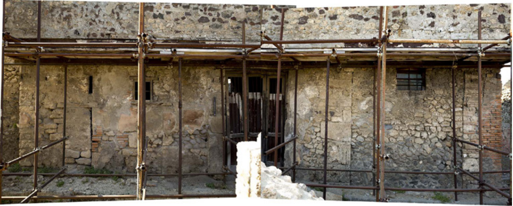
Figure 6. Pompeii, Regio VII, insula 12: the facade of the Casa del Balcone Pensile (VII, 12, 28). On the left, the buffered doors of number 29 (Photogrammetry by 'Great Pompeii Project'. Topographic Referent: P VII 12 S3. Licensed by the Ministry of Culture - Archaeological Park of Pompeii: reprints or duplicates are forbidden).
